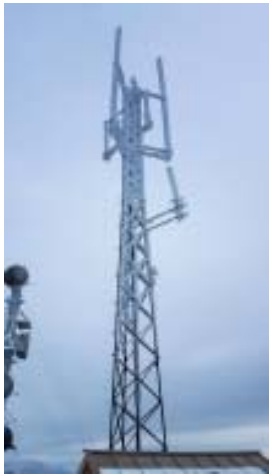
Just a little bit of ice build up on the tower and antennas.
