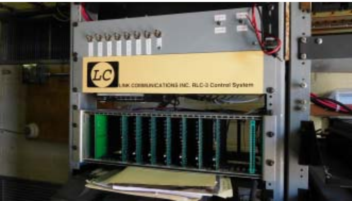
RLC-3 Link Communications controller with power switch panel above and radio card cage below.
