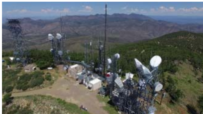
Aerial photo of Mt. Ord site. ARA building and tower is to the left of the red truck.
