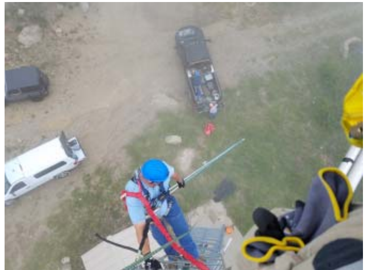
At Pinal Peak, tower climbers wait for the replacement antenna to be hoisted up.
